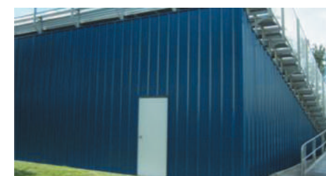
Metal Panel Enclosure
